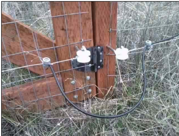
Figure 5. Black-colored insulated electric fence wire, 12-gauge. Used here to connect the electrified lines of a gate to the main electrified lines on the fence.
